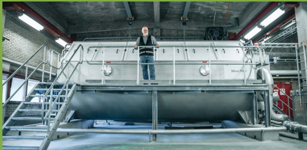
The new filtration system weighs forty-two tons and measures about thirty-three feet long by ten feet wide by ten feet high.
